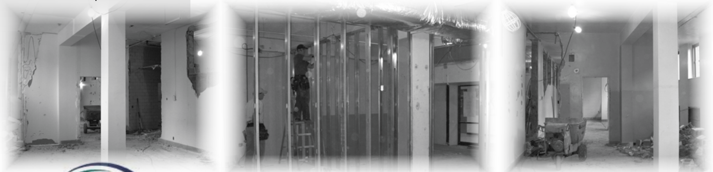
The Clinical Nursing Resource Center is under construction and scheduled for courses in January.
