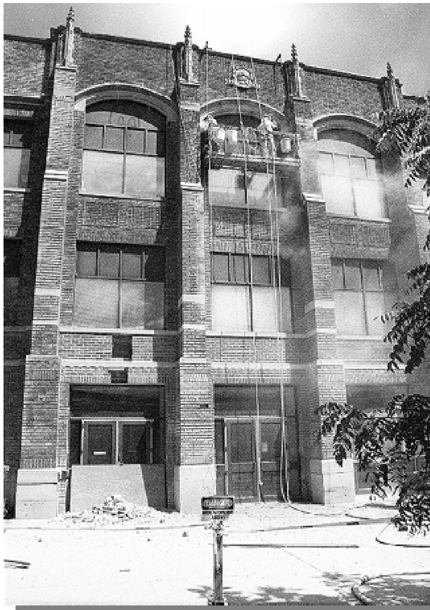
The 90-year-old Deputy Hall received a much needed facelift this summer when workers removed and replaced the mortar between the bricks.
