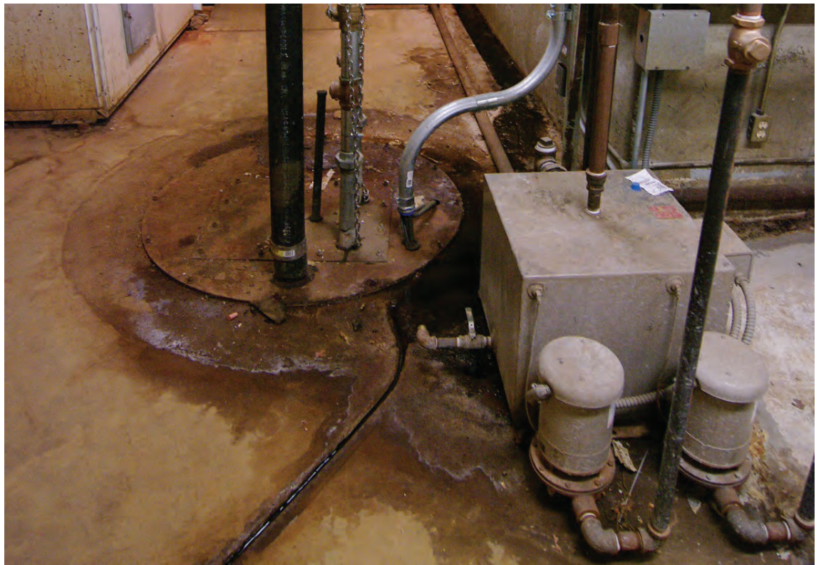
sump in basement constantly draining water
