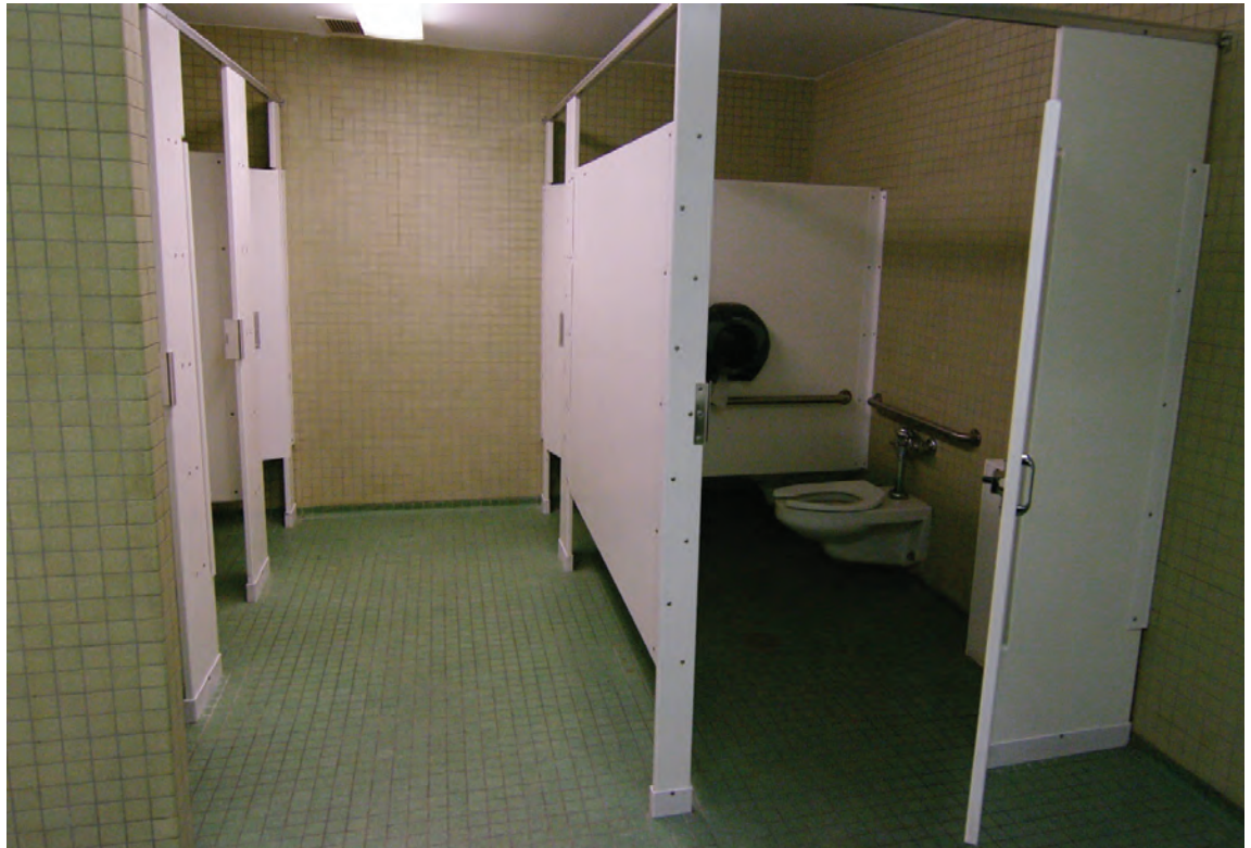
typical non-ADA compliant stall
