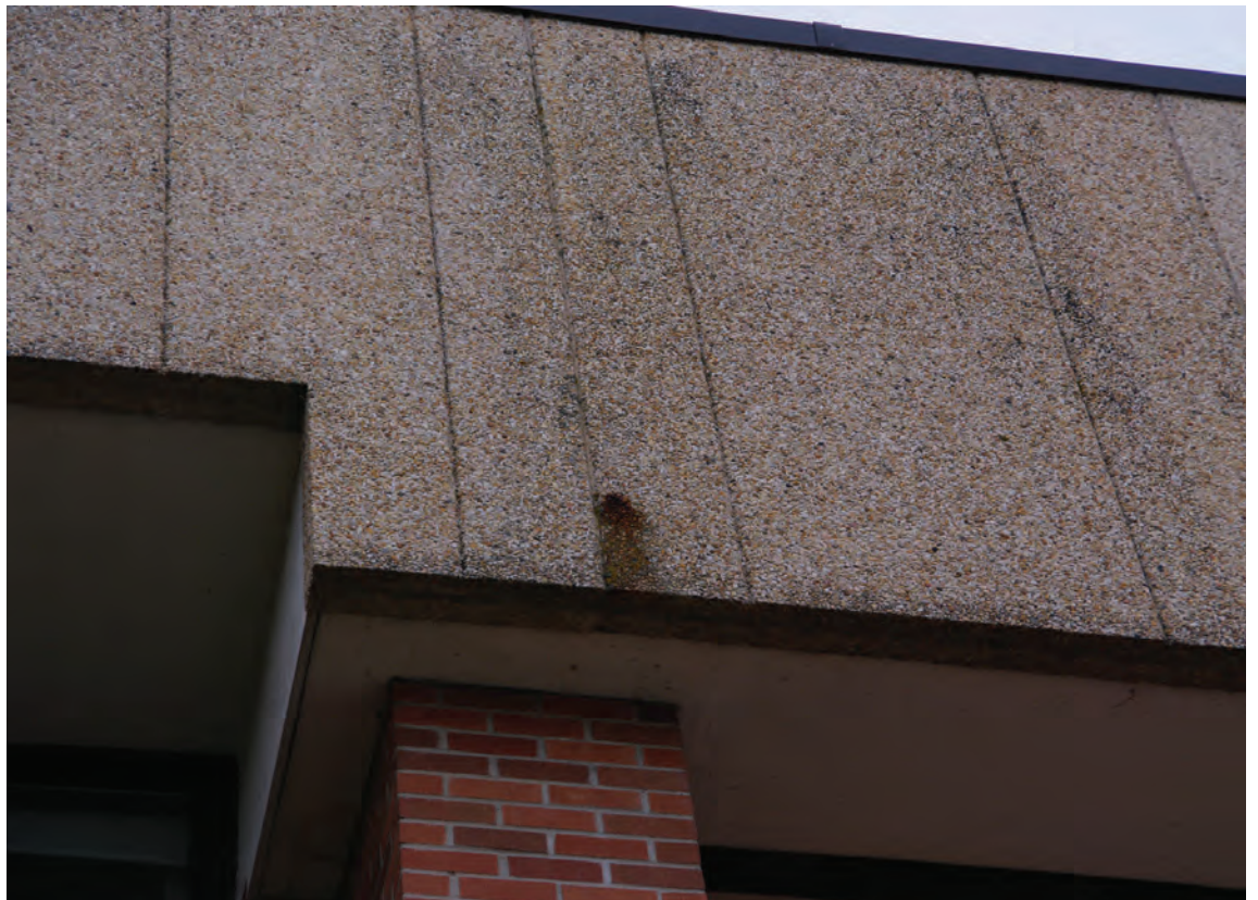
rust and dirt stains on precast concrete
