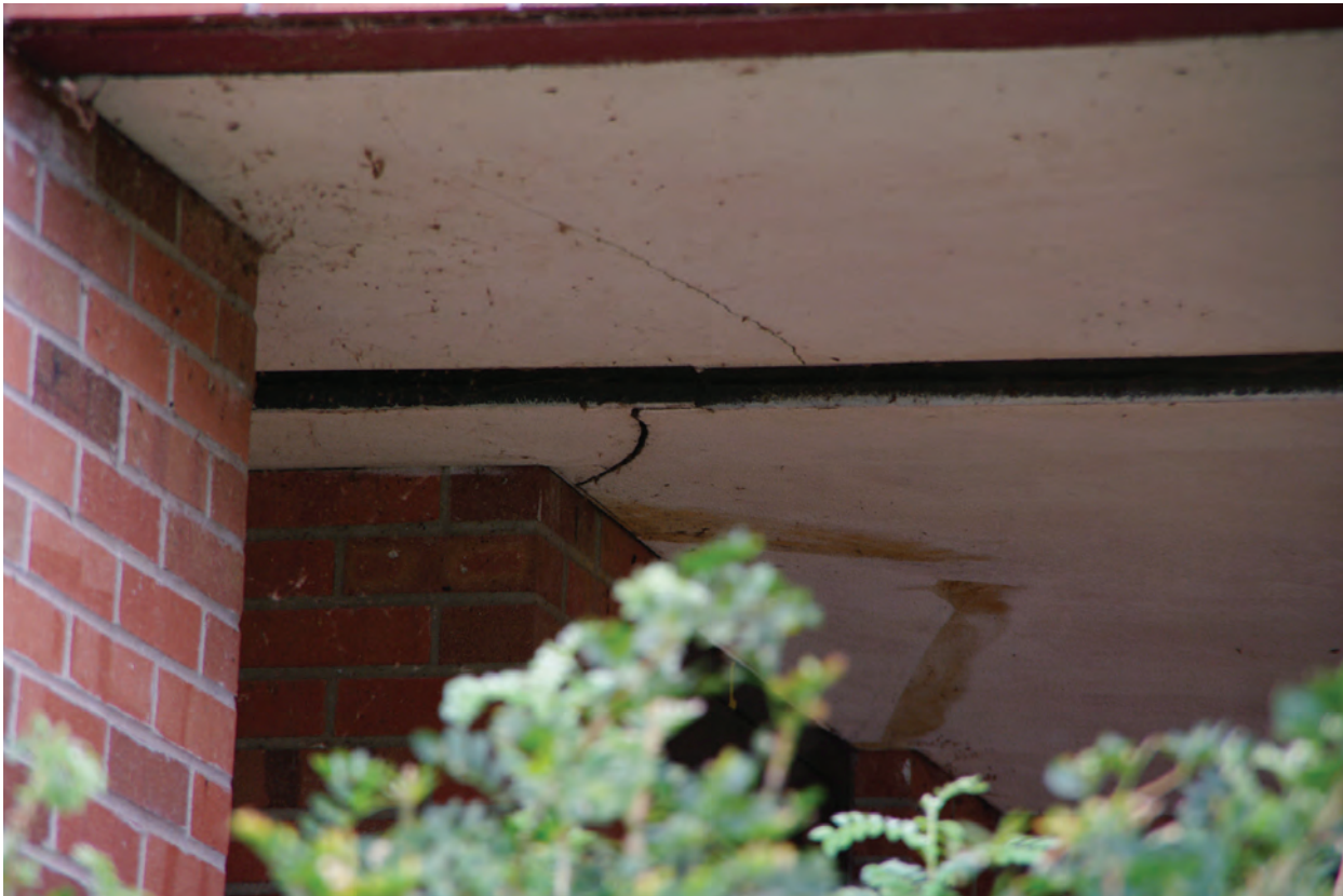
cracks in exterior first floor soffits
