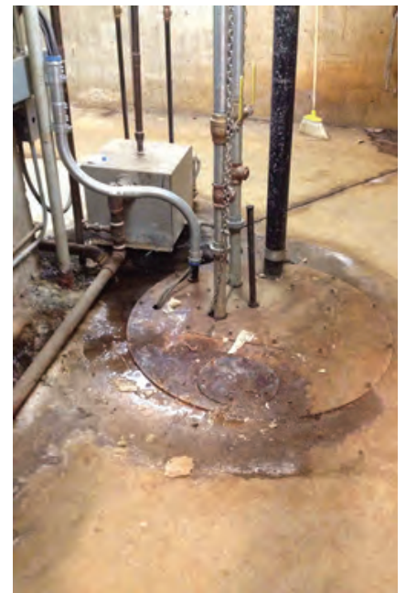
current sewage ejector pit
