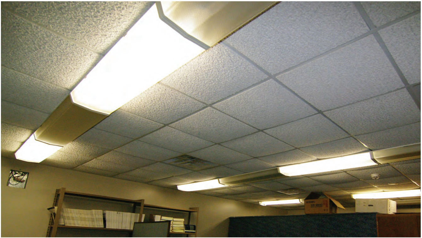
sagging ceiling tile
