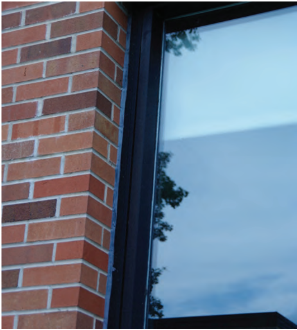
uneven gap between sash and frame
