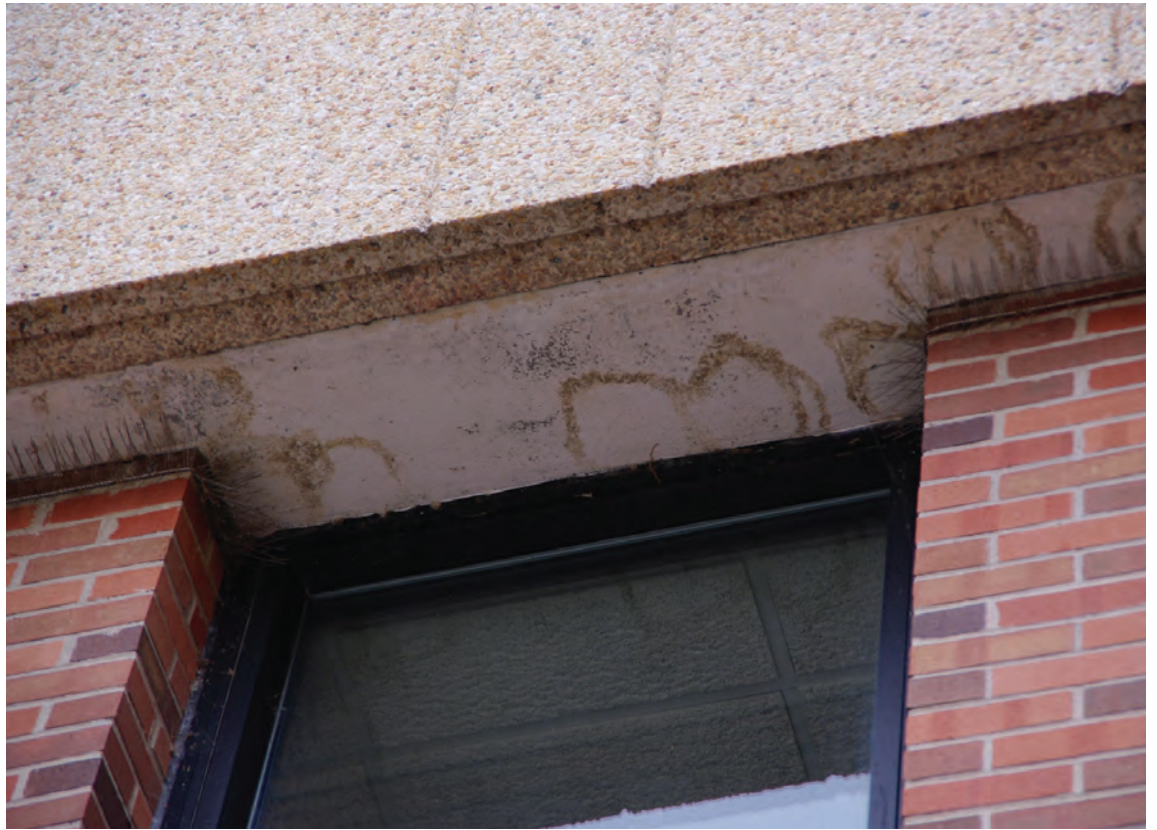
staining at soffits
