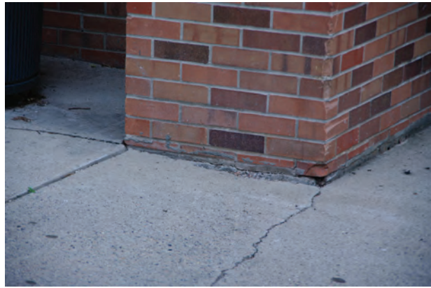
chipping on brick corner
