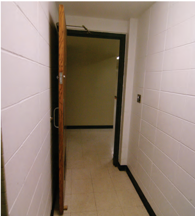
non-ADA compliant door at restrooms
