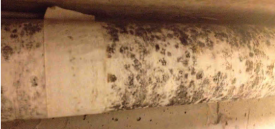
Mold in Tunnel Space
