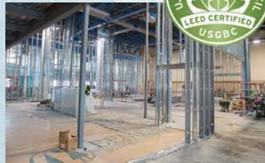
Renovated Memorial Hall, under construction in this Jan. 2015 photograph, is LEED-certified for energy efficiency.
