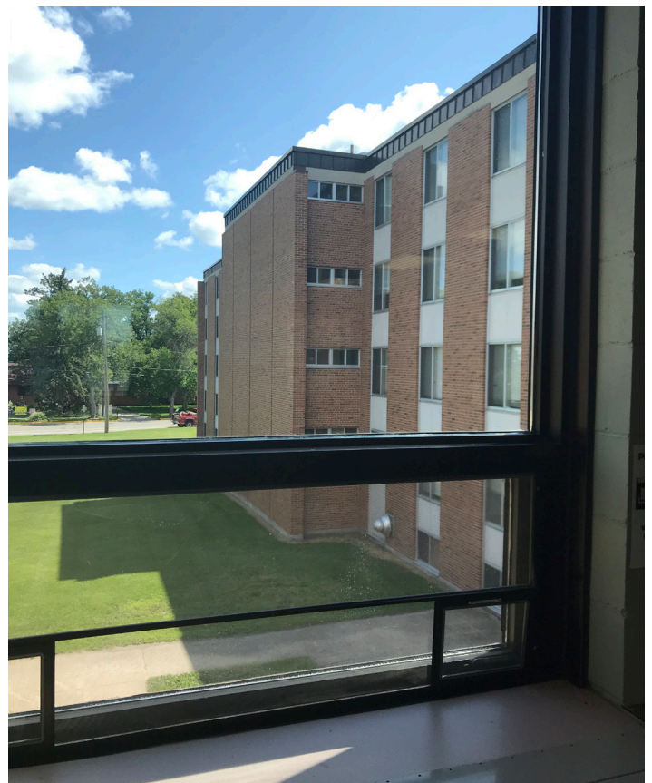
RIGHT: Residential buildings have substantial amounts of deferred maintenance which lead to higher operational costs and decreased comfort for students, but the funding for renovations needing to come from Revenue Bonds and not General Obligation Bonds makes it more difficult to finance renovation or new residential projects.
