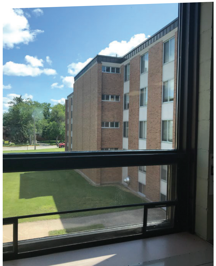
RIGHT: Residential buildings have substantial amounts of deferred maintenance which lead to higher operational costs and decreased comfort for students, but the funding for renovations needing to come from Revenue Bonds and not General Obligation Bonds makes it more difficult to finance renovation or new residential projects.
